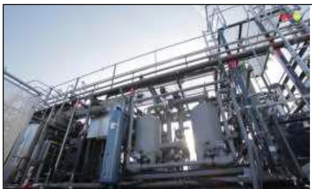
Fig. 3 Cryo Pur bio-LNG demonstration plant at Valenton Waste Water Treatment Plant.
