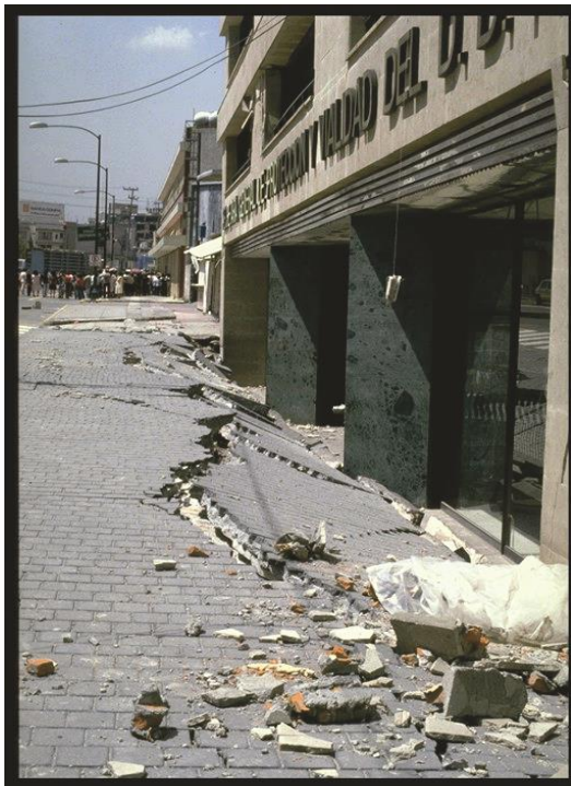
Fig. 1 Settlement of a building at Mexico City during 19 September 1985 Michoacán earthquake.
