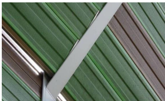
Fig. 4 Insufficient supporting of the panels on the inclined part of the noise barrier.
