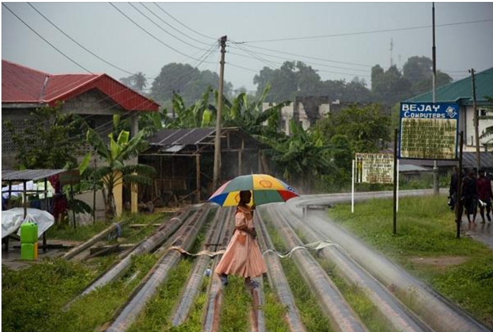
Fig. 2 Erosion exposes Oil pipelines in a community of Okrika. Source: Circles of Blue, 2009.
