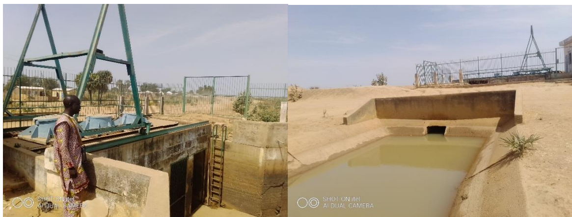
Figure 3. Pumping station and drain station water pipeline.
