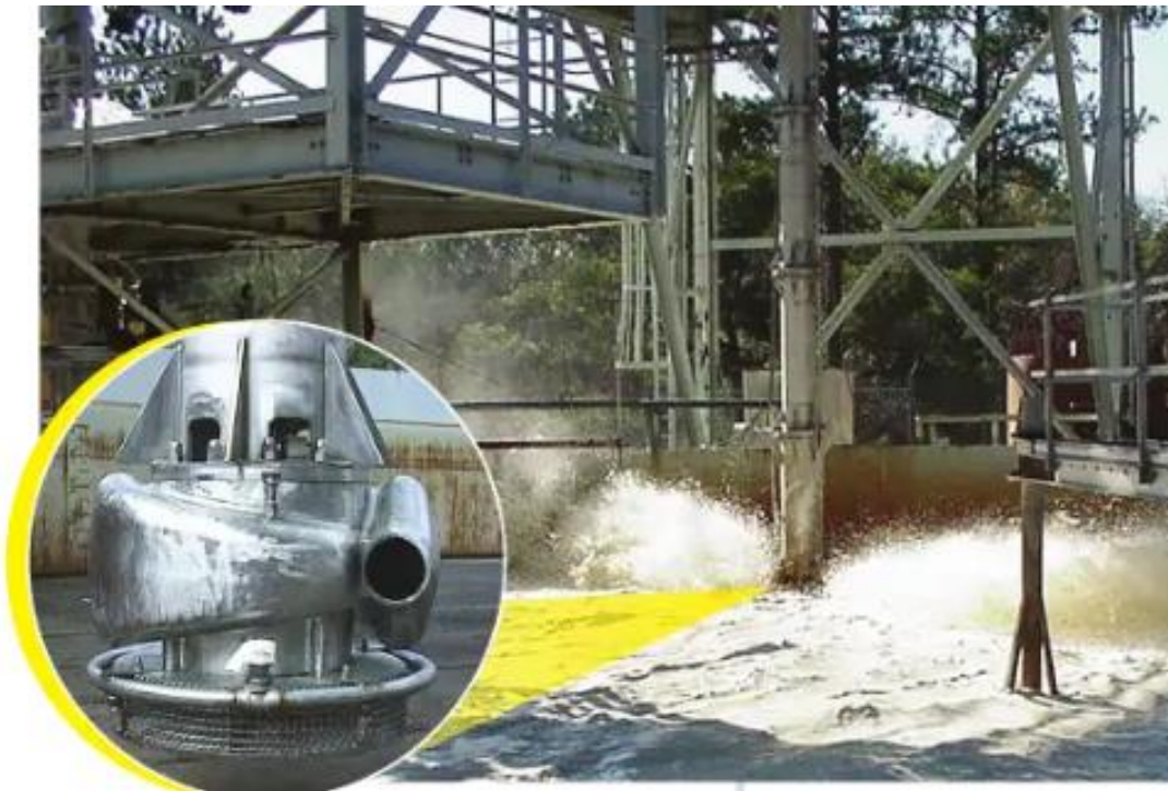
Figure 1. A 1.3-million-dollar mixing pump at Savannah River Site.
