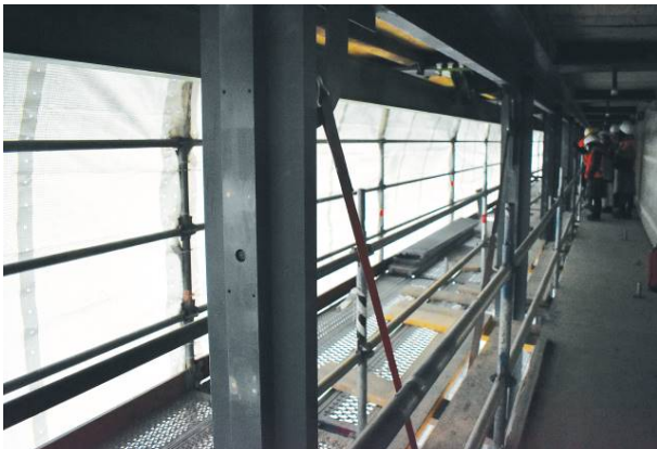
Fig. 5 Restoration site of the Neue Nationalgalerie, cross-bracing reinforcements to reduce deformation of steel components (Di Resta 2019).
