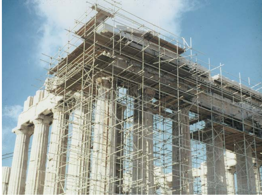
Fig. 3 The south east part of the Parthenon under repair some years ago.
