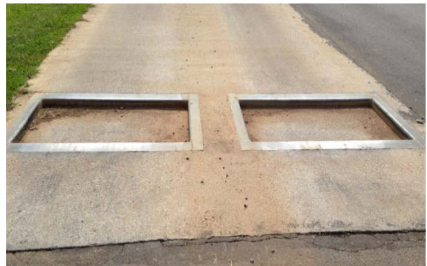
Fig. 9 Detail of the pothole track.
