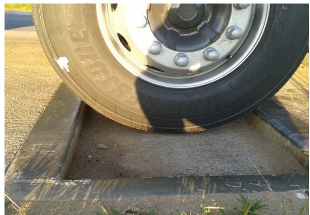
Fig. 10 Interaction between tire and pothole.
