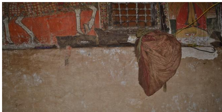
Figure 3. Mural painting damaged by flood (Qoma Fasilads).
