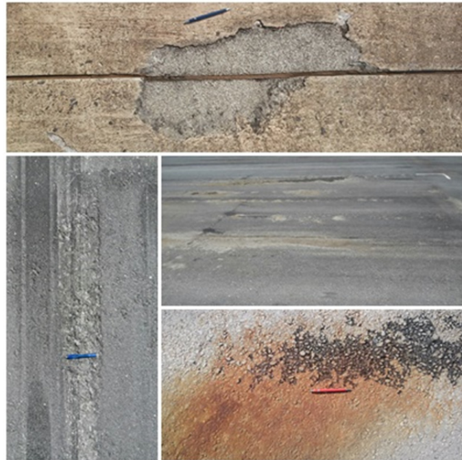
Fig. 4 Airfield distress in the study, weathering, and cracking.
