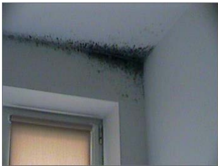
Fig. 7 Exemplary detected troubles in the tested residential apartment buildings: mold in the room corner, on the internal surface of the external wall.
