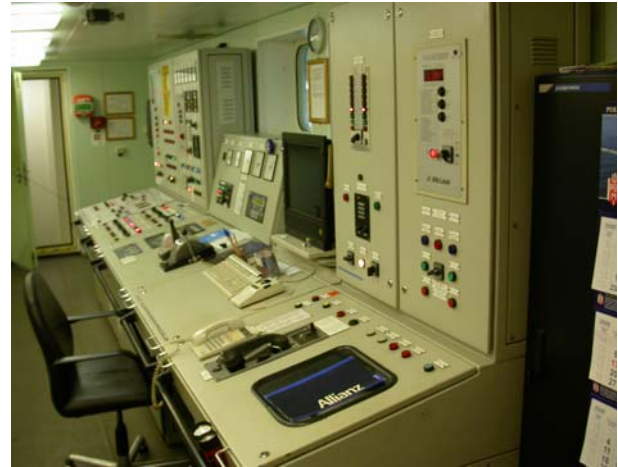
Fig. 6 View of a manoeuvring-controlling centre.
